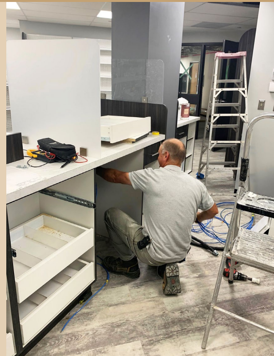
Final work on the construction of the new Pharmasave outlet was completed in mid-September.
